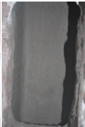
Duct after treatment.
