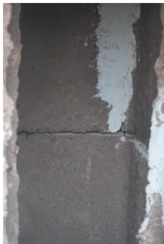
Duct before treatment.
